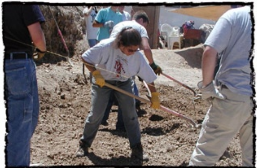
Day 2: Presytera Becky takes shovel in hand to level out the ground. The Project Mexico staff said this property required more moving of dirt than any previous site.
