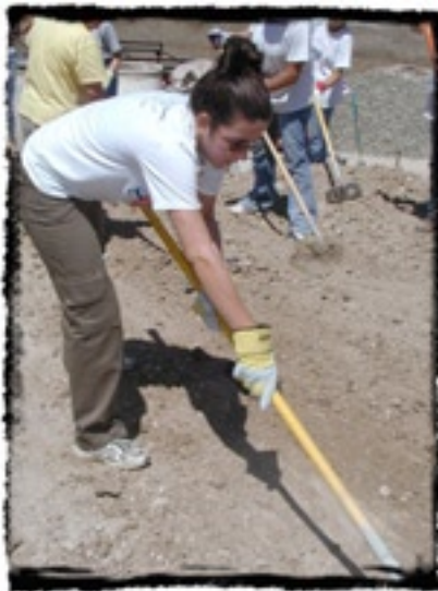
Day 2: Eleni Valliant tills the ground as the team prepares the soil for the foundation of the house. Only hand tools are used.
